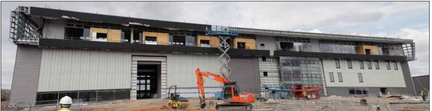
The size of a football pitch: the Nuclear AMRC's main research facility on the Advanced Manufacturing Park, South Yorkshire, July 2011.
